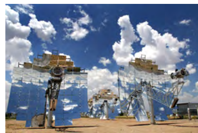
Figure 5. Stirling dish engine. These beautiful concentrators deliver a power per unit land area of 14 W/m 2 . Photo courtesy of Stirling Energy Systems. www.stirlingenergy.com
