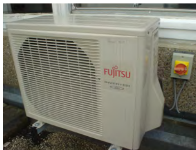
Figure 13. Good: The inner and outer bits of an air-source heat pump that has a coefficient of performance of 4. The inner bit is accompanied by a ball-point pen, for scale. One of these Fujitsu units can deliver 3.6 kW of heating when using just 0.845 kW of electricity. It can also run in reverse, delivering 2.6 kW of cooling when using 0.655 kW of electricity.
